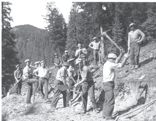
WWII COs building road in Jasper (Alberta) national park. CMBS, Winnipeg. John M. Schmidt collection.
